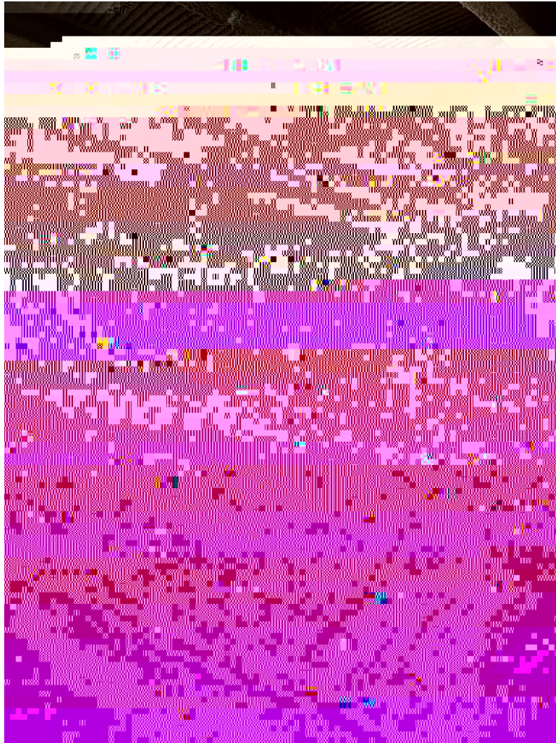
Preparation for Small Venue CMU wall installation. Weather wall installation at Ground Level has begun.
